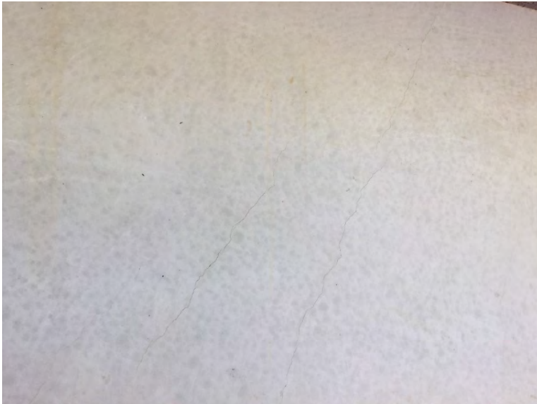
Hairline cracks noted on upstream girder
