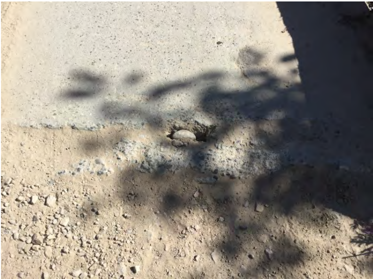
Damage to top of right bank ballast wall and deck panel 1
