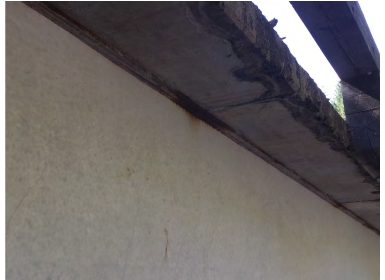
Evidence that water has been getting through deck joints
