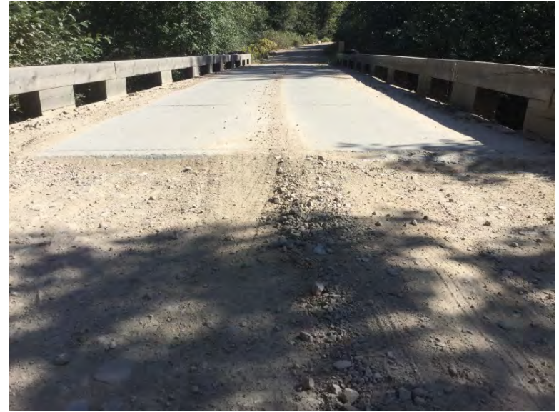
Bridge deck sits higher than road surface causing damage to ballast wall and deck panel at right bank
